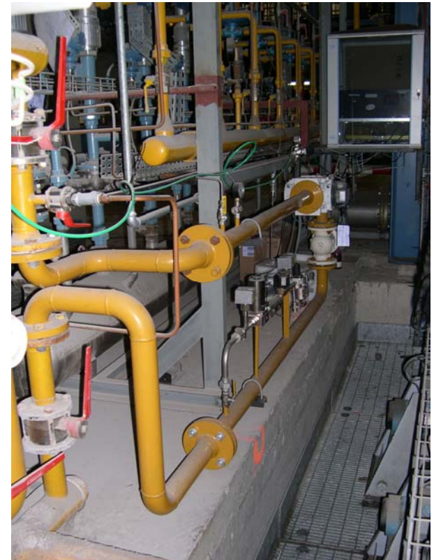
Example of INDELIS installed in glass industry for supplying feeders
