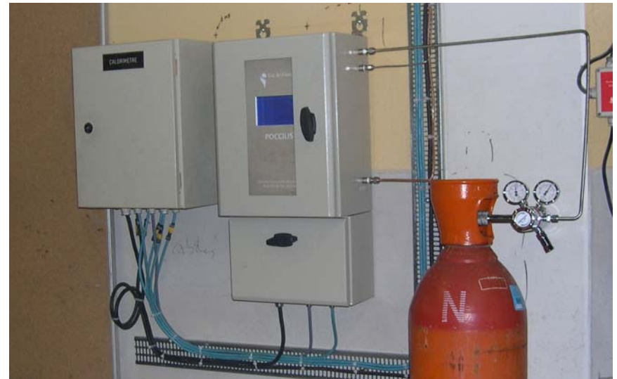
POCCILIS installed at a bottles manufacturer
